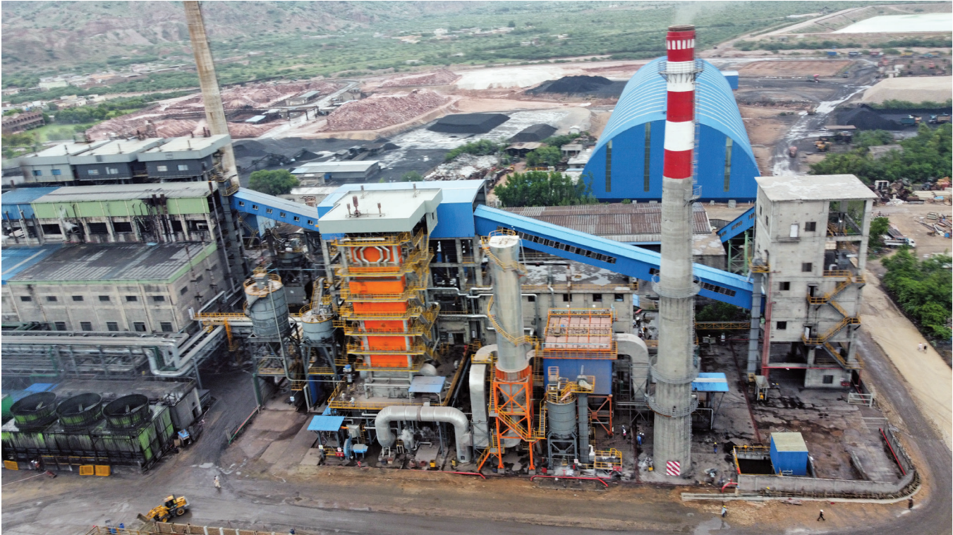
The Soda Ash Business installed and commissioned a biomass feeding system at its plant as part of the Coal-Fired Boiler project.
