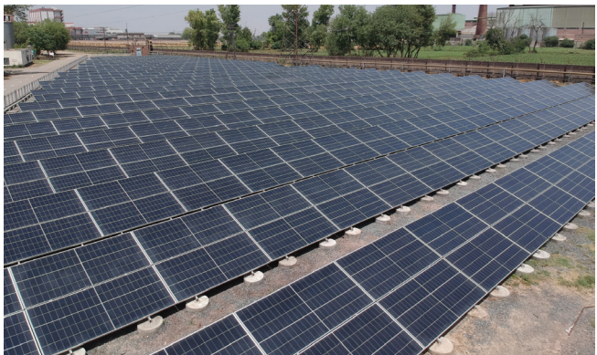
The Polyester Business commissioned a 1 MW solar power system at the Polyester Plant, Sheikhupura.
